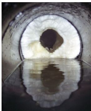
Figure 1: Hydrate in a Pipeline.
