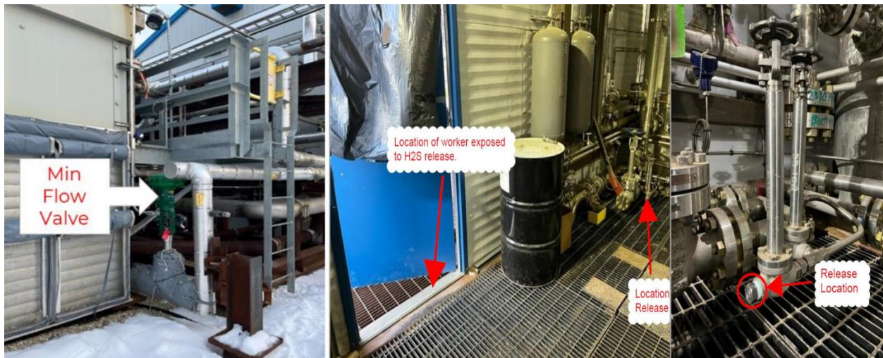
Left: Valve outside being worked on. Middle: Location of worker exposed to H 2 S. Right: H 2 S release location.
