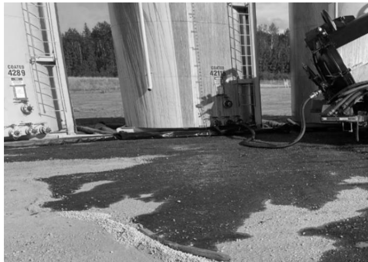
View of Spill at Slop Tank
