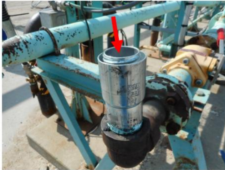
Hose separated from the crimped fitting
