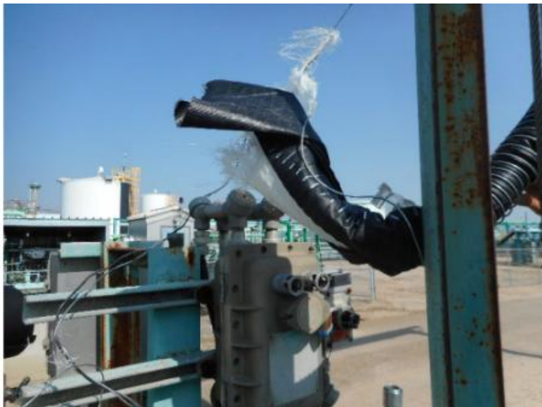
Hose condition in location after the event
