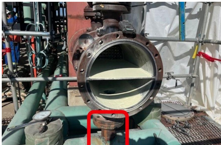
Image: View of leak on exchanger
