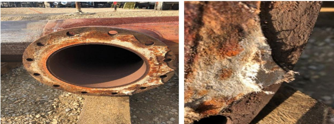
Images: Stack flange face showing asbestos gasket
