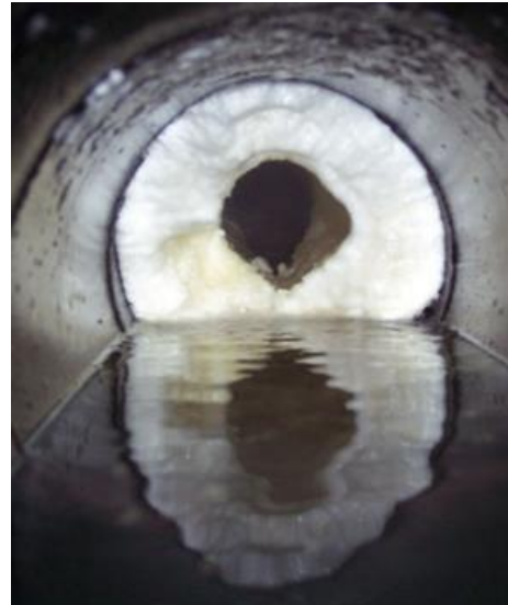
Figure 1. Hydrate in a Pipeline
