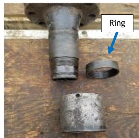
View of connection that failed, including ring
