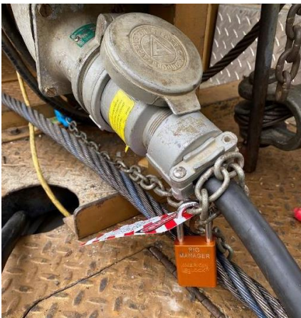
View of proper power cord lockout
