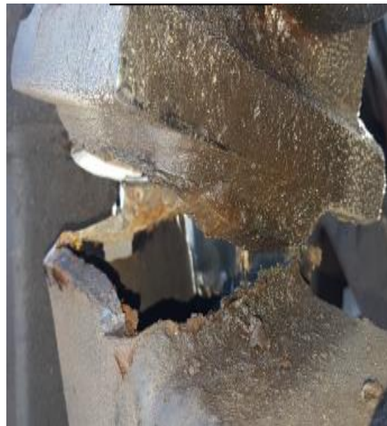
Driller side bracket. Close-up view of cracked mast.
