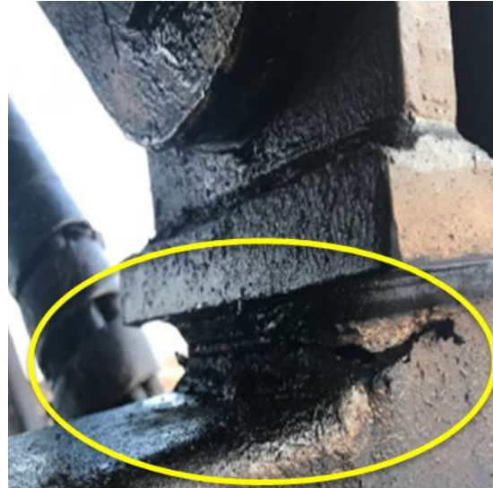
Off-driller side bracket cracking.
