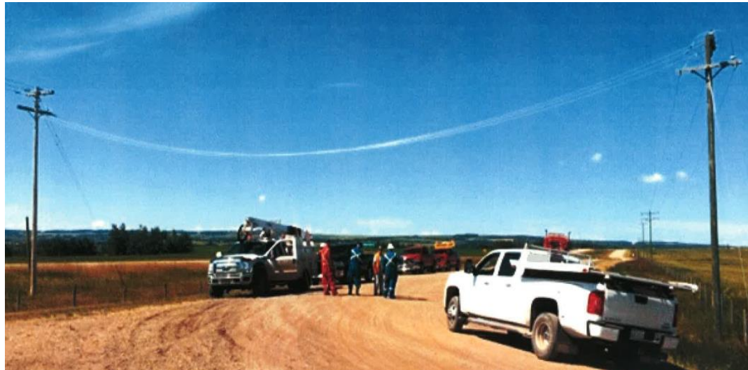
A windstorm the night before caused a power pole to shift and the overhead powerline across the road to sag
