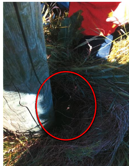
The hole in the ground shows that the pole shifted significantly in the windstorm
