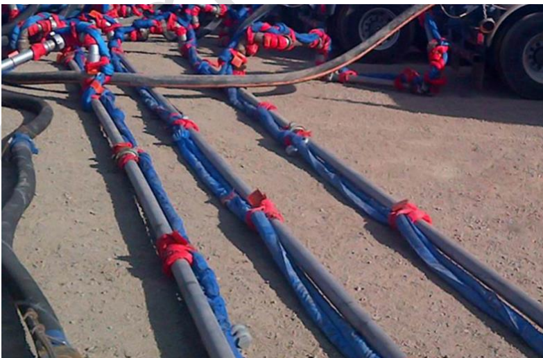
Figure 38. Anchor Line Tie-Off Restraint System (Spine and Rib)
