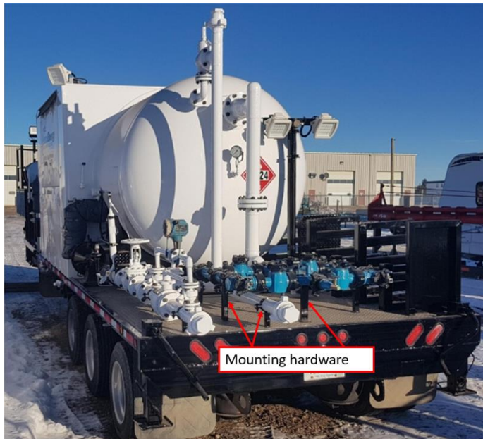
Figure 30. Example of Mounted Pipework
