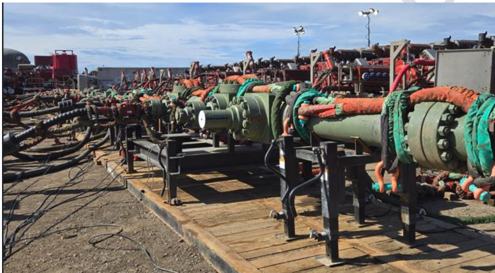
Figure 40. Large Bore Fracture Pipe Restraint
