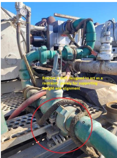
Figure 34. Fracture Pump Bracket
