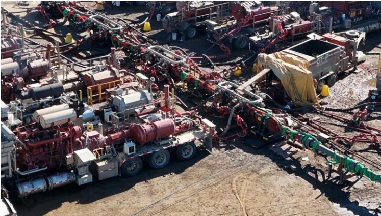
Figure 6. Discharge Iron from Fracture Pumps to Manifold Trailer with Restraints
