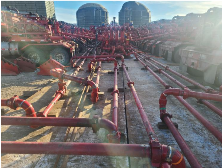
Figure 2. Hydraulic Fracturing Pipework System Before Restraint Application
