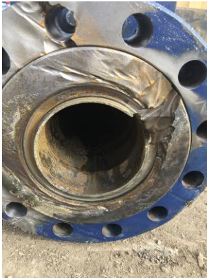
Figure 26. Example Flange Failure
