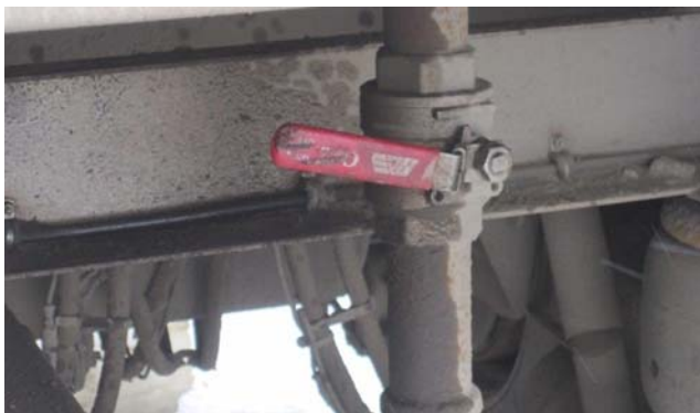
Drain valve that was left in the open position
