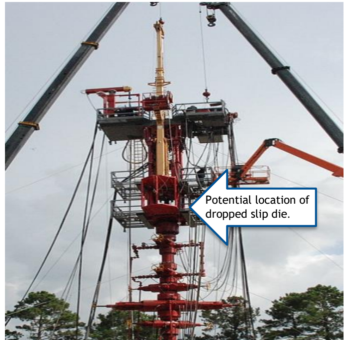
Typical stacked snubbing rig
