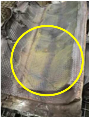
Chromium residue on insulation
