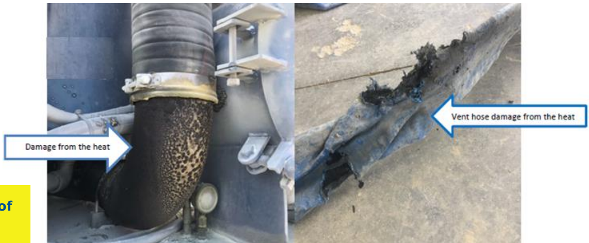
CLOSE-UP OF HOSING FAILURE
